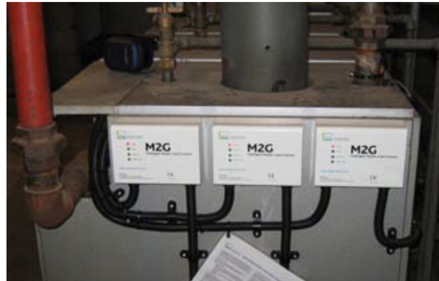
3 boiler load optimisers controlling 3 boilers
