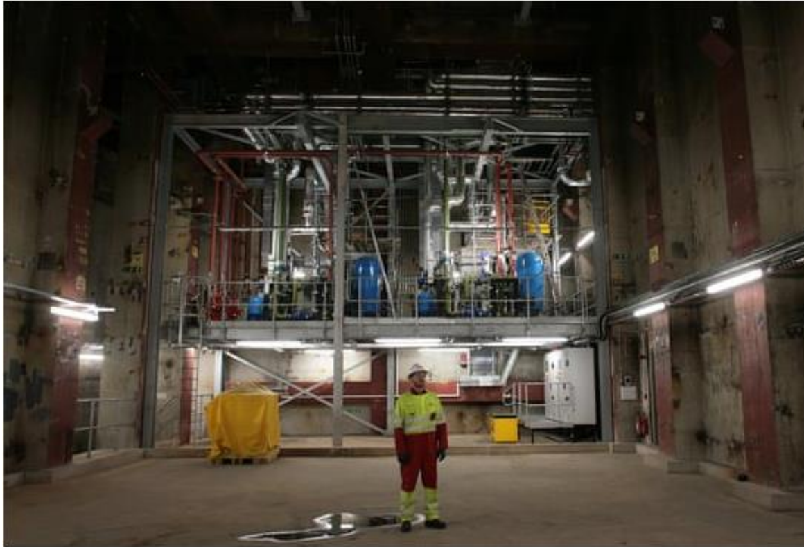
Old CHP Engine Bay
