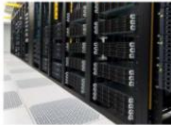
Data Centre and Mission Critical
