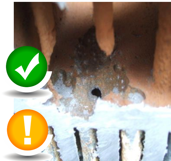
Heat exchanger after a few months
